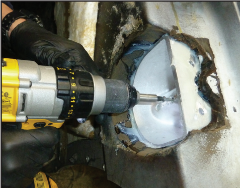
Install the plug & use a #10 wood screw to secure the plug in position. Wipe up excess adhesive with a gloved finger or spreader.
