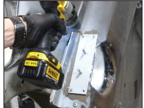
With a rivet temporarily placed in the first hole as a guide, drill the remaining rivet holes. Remove the plate, bolts, and rivet.
